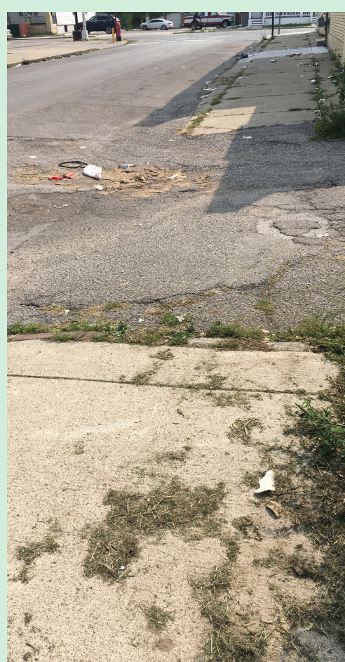
Issues with Alley crossings in Hamtramck
