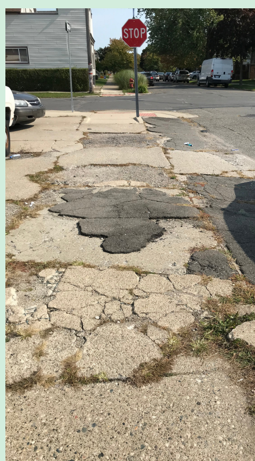
Cumblng sidewalk in Hamtramck
